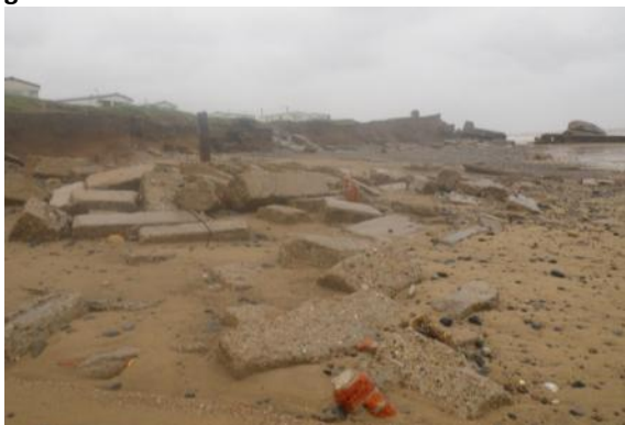
Photo 16 Sections of the old seawall and brickwork rubble, south of the southern 9.2 inch gun apron
