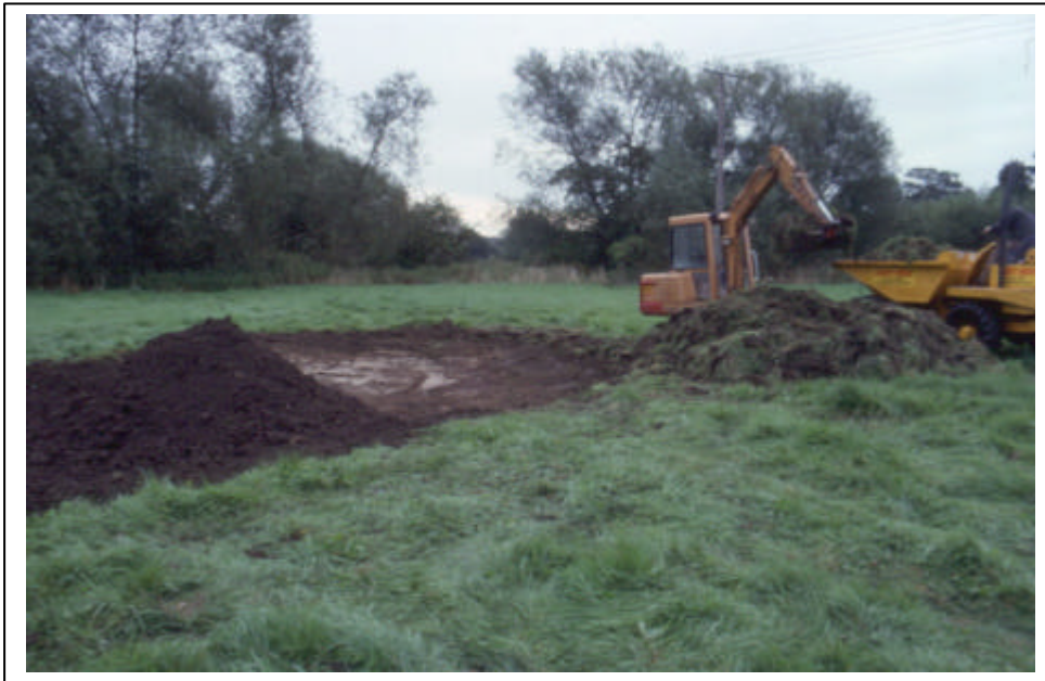
Photo 2.15. Langel Common, Witney, restoration site. Constructing the scrape, subsoil and turf at right to be removed; topsoil heaped at left to be re-spread. Photo by C.R. Lambrick.
