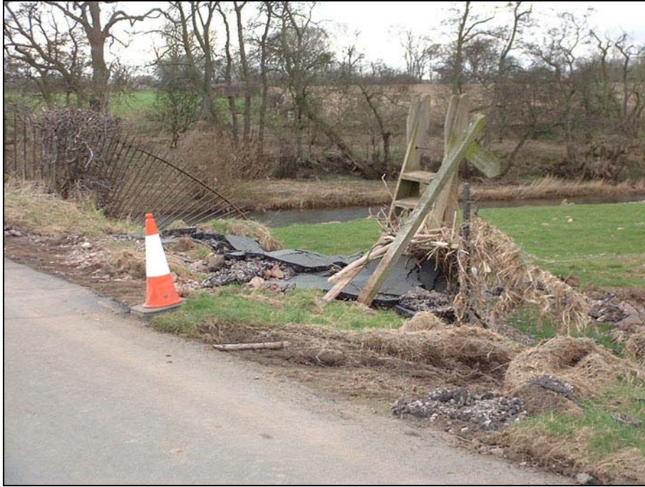
Damage on the Caldew
