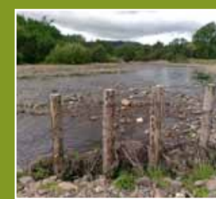
River bank erosion
