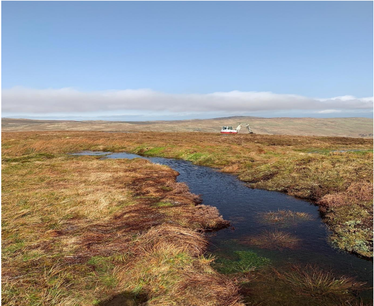
Newly constructed horseshoe bund on upland blanket bog, above Shap, Cumbria. Photo: Deborah Land, Natural England
