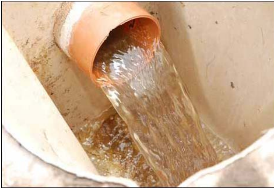
Figure 2.3 Clarified effluent from a septic tank.
