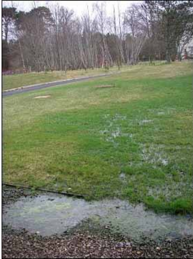
Figure 2.4 Effluent discharging onto the soil surface as a result of hydraulic failure in a septic tank system; note the algal bloom that is developing on the nutrient rich puddle that is forming at the base of the slope.
