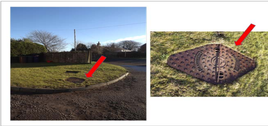
Plate 2 Location and sampling point for Tank 2, showing the location of the cover that provided access to the inspection chamber
