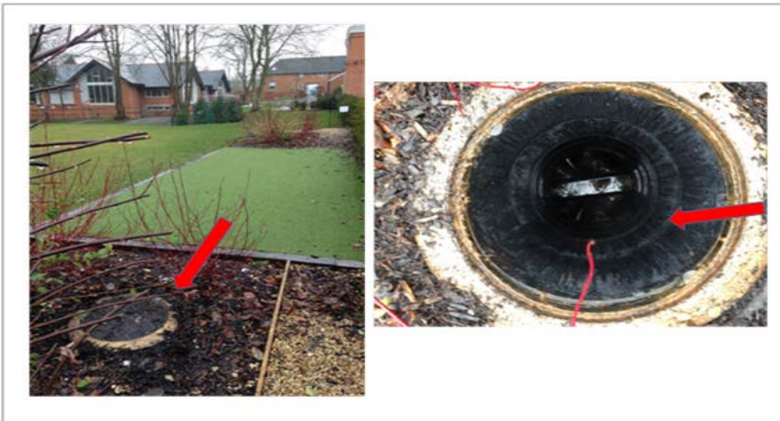
Plate 4 Location and sampling point for Tank 4, showing inspection cover and effluent sampling point within the inspection chamber
