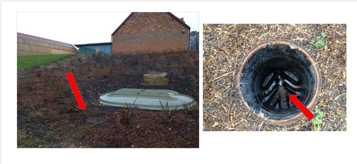
Plate 6 Location and sampling point for Tank 6, showing inspection cover and effluent sampling point within the inspection chamber
