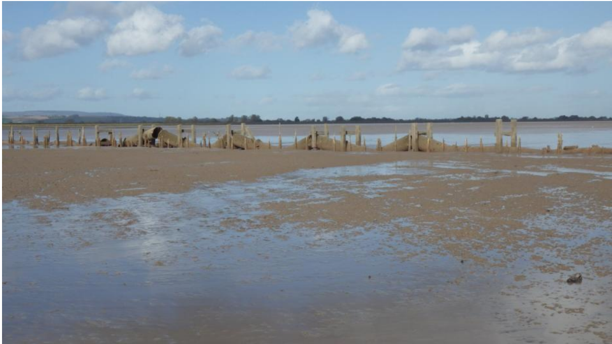
Plate 10. A large disused outfall on the Peterson Flats between Newport and Cardiff
