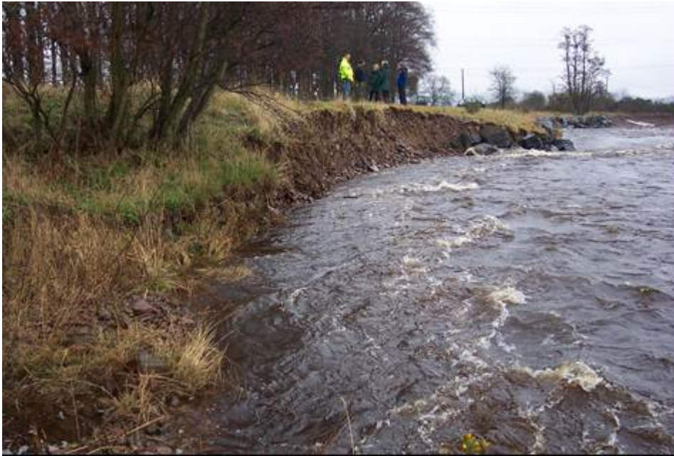
Figure 2.19 Bank reinforcement aimed at preventing lateral channel movement, but actually exacerbating bank and bed destabilisation
