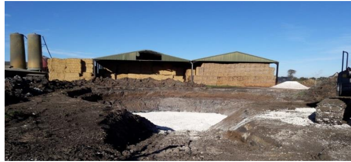
The photograph above shows the groundworks of the site which will house the sulphuric acid tank, and mixing and pumping chamber.
