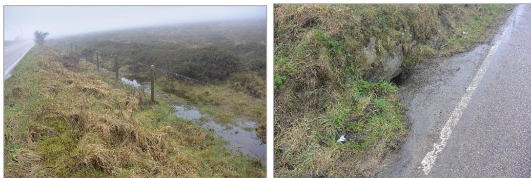
Figure 3.3-1. a) Moorland upslope of the South-eastern Area and B3318, with water ponding against the road after significant rainfall, and b) roadside culvert allowing runoff from the road into the site.
