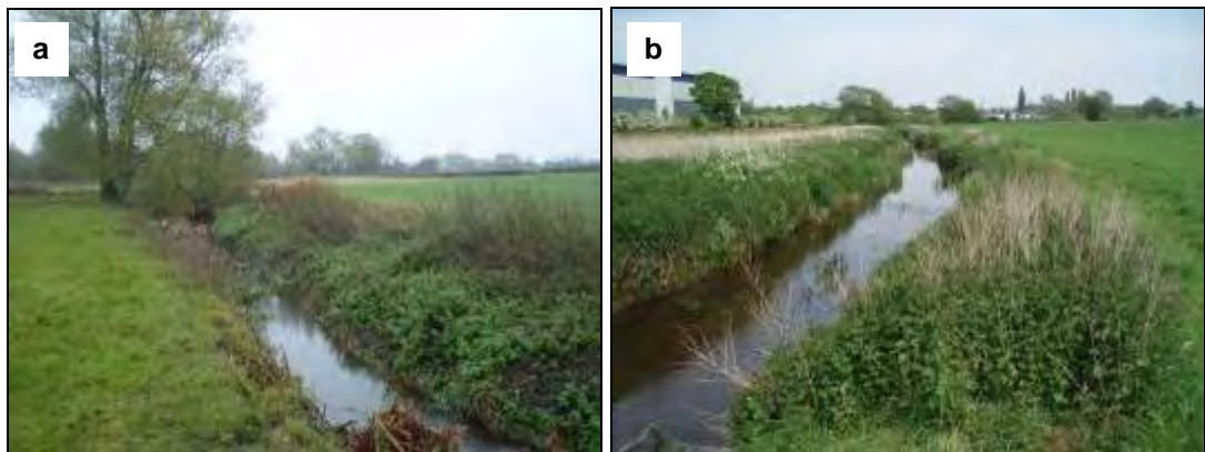
Figure 5.9: Examples of sections of channel with uniform cross-section indicative of past re-sectioning (a) reach MEA002 and (b) MEA005 (Photograph b courtesy of the Environment Agency)
