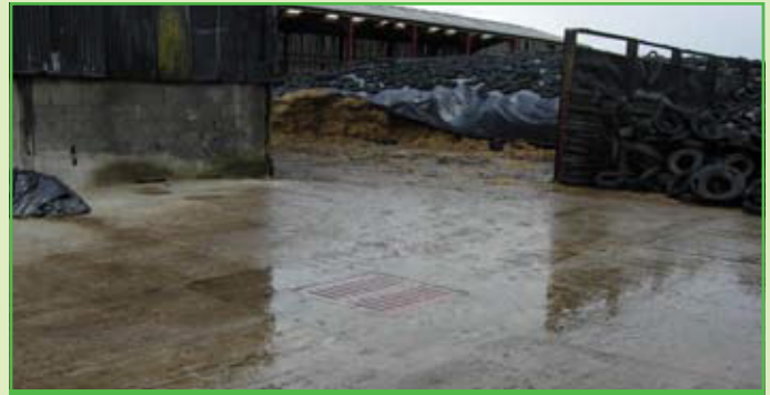
Part CSF funded concrete yard with drain to divert foul water to slurry lagoon
