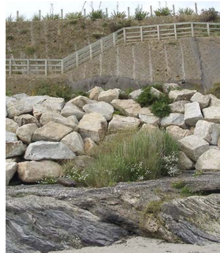
The sequence of Quaternary sediments resting on the raised wave-cut platform at Gerrans Bay SSSI, Cornwall. Here, rock revetments and concrete walls have been used to protect the cliff from erosion and failure due to wave action, with the consequence that the sediments are effectively inaccessible along this portion of the site. ©Natural England/Natalie Bennett
