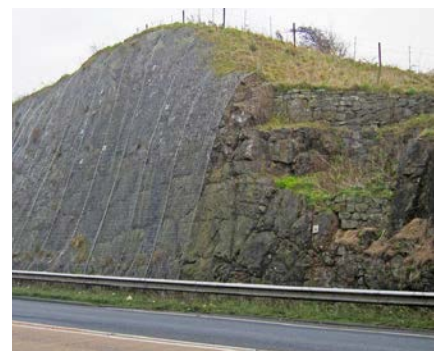
Road cutting on the A690 north of Dalton-in-Furness, Cumbria. Rock fall netting can have severe impacts on both visibility and accessibility of geodiversity, promoting vegetation growth behind the netting. ©Natural England/Dave Evans
