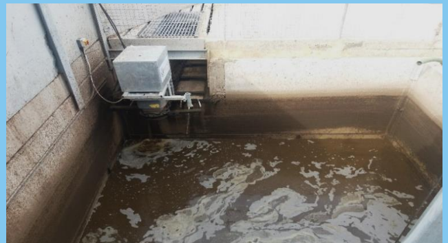
Reception pit with chain driven channel conveyor.
