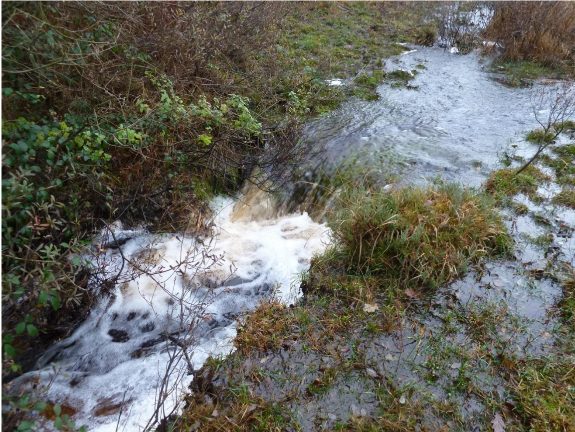
Figure 1-10: Knick point erosion in downstream stream section
