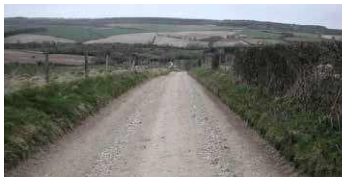
Before work commenced; showing the extent the track had to be raised.
