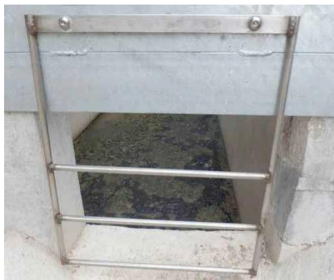
The sediment trap overflow outlet showing the solids trapped since installation
