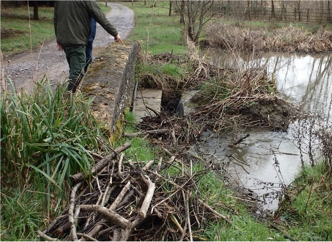
Figure 7. Dam at a track culvert resulting in some management issues. © A. Rothwell
