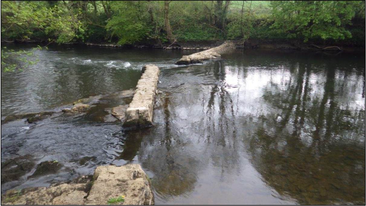
Figure A49. SX4138773683. Double fishing croys. Potential barrier to shad. Viewed from Devon bank looking downstream.
