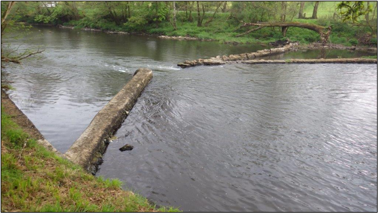
Figure A47. SX4147373352. First weir immediately upstream of Duchess Weir, adjacent to Weir Cottage. View from Devon bank looking downstream.
