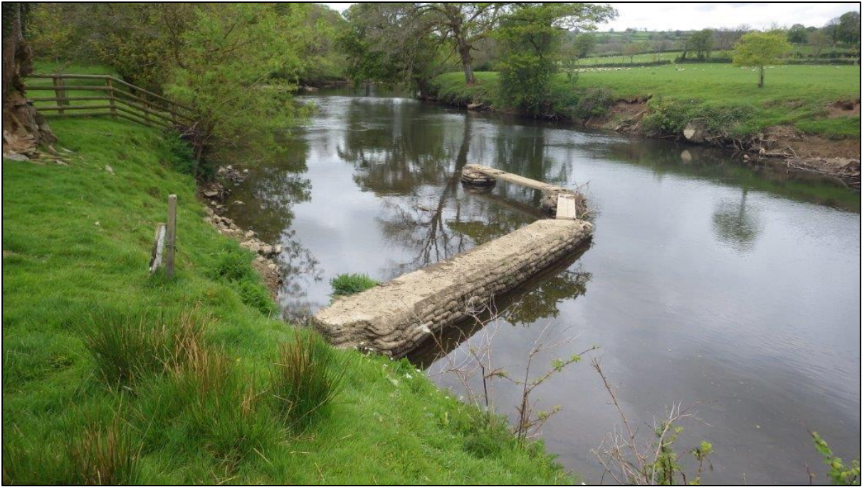
Figure A79. SX3994874036. Fishing croy and platforms on Devon bank. Viewed from Devon bank looking downstream.
