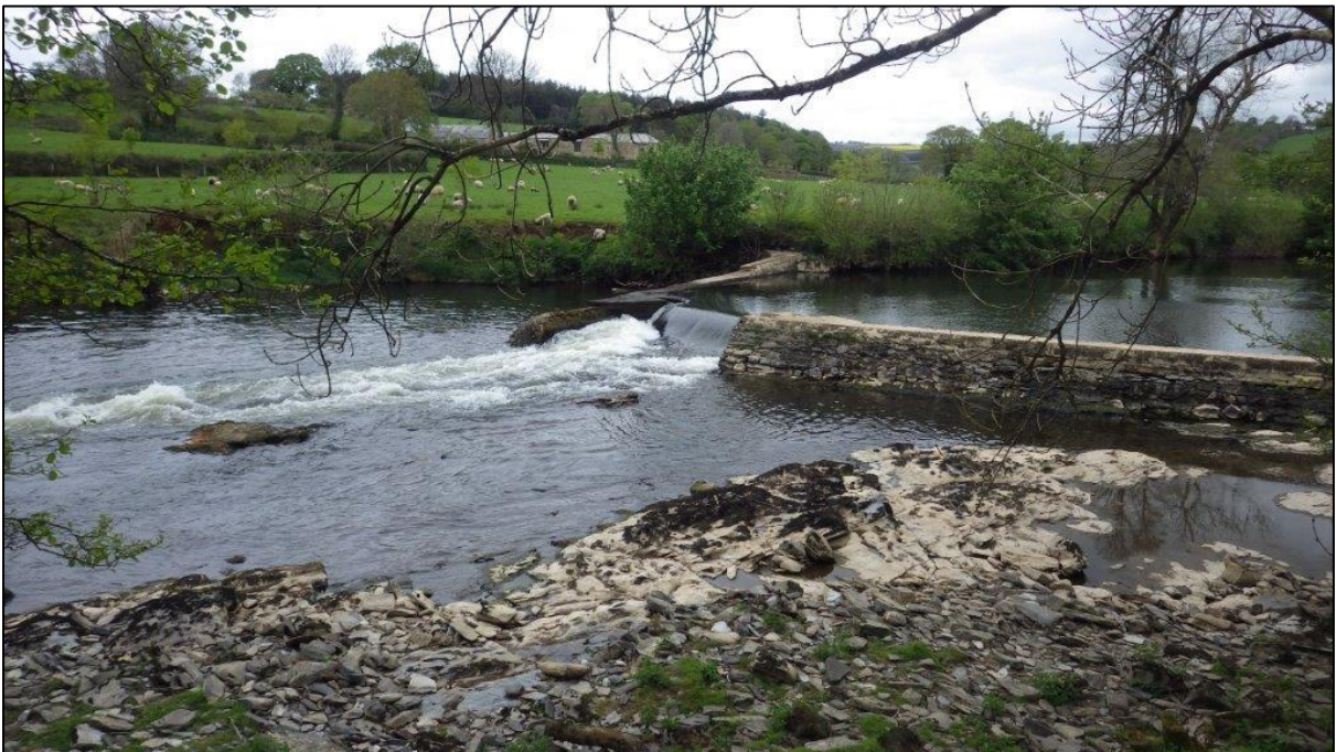
Figure A76. SX3962073940. Lamerhooe Weir and bedrock on Devon bank. Significant barrier to shad. Viewed from Devon bank.
