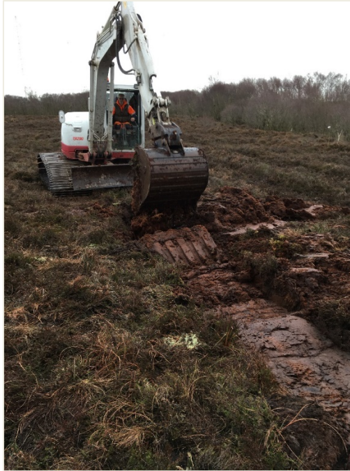
Picture 4.5 Earthworks during peatland restoration at South Solway Mosses, Cumbria. © Natural England / Ian Crosher
