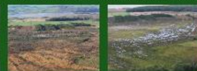
Roudsea Wood and Mosses SAC Bund and cell construction on degraded lowland raised bog
