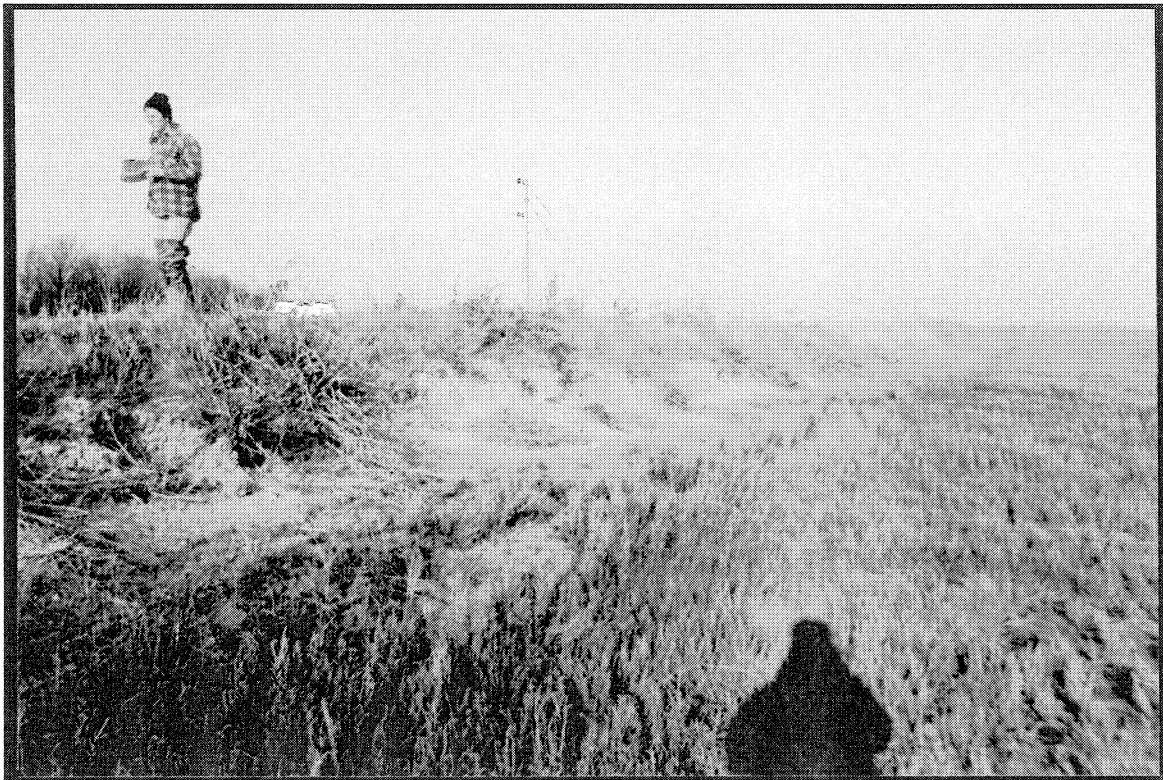
Plate 12: February 1994 Closer view of erosion of the inner sea wall
