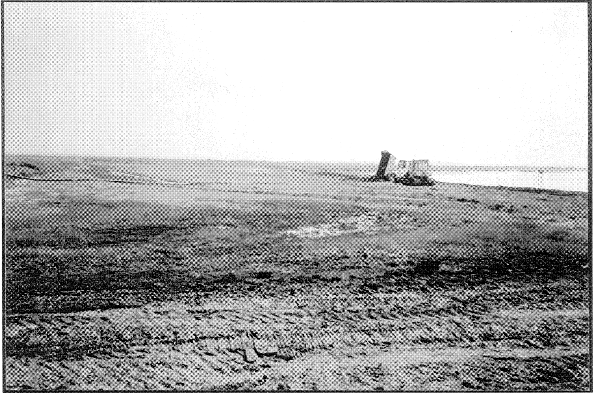
Plate 7: June 1992 View looking east across site during maintenance work to infill the borrow pits
