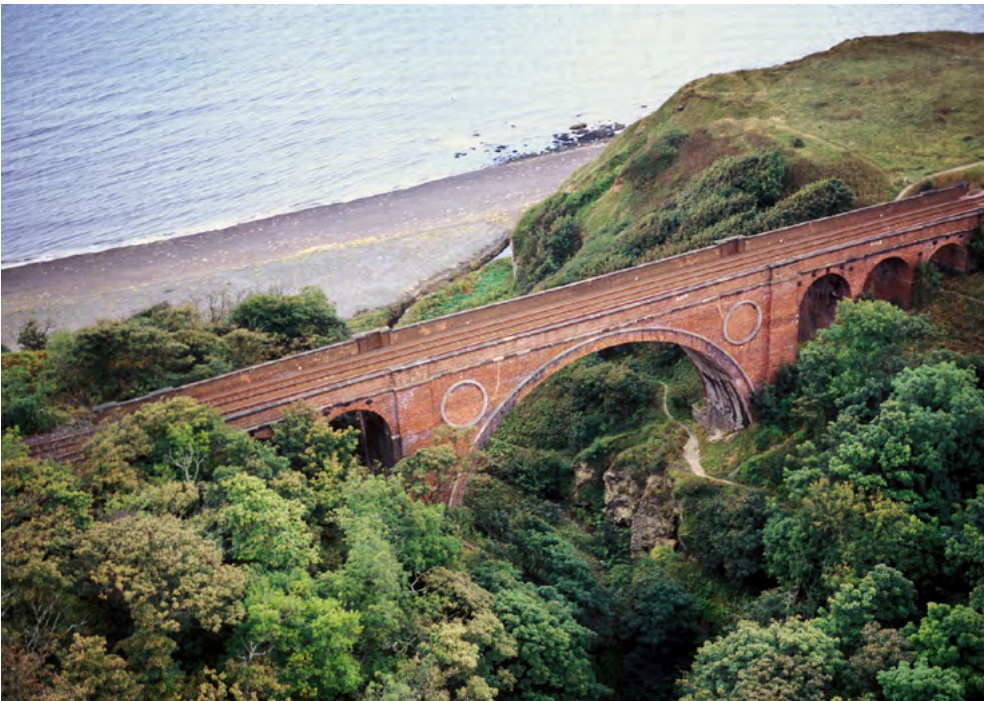
Hawthorn Dene, and the other coastal denes, safeguard valuable fragments of ancient woodland and often have historic transport structures such as this viaduct.
