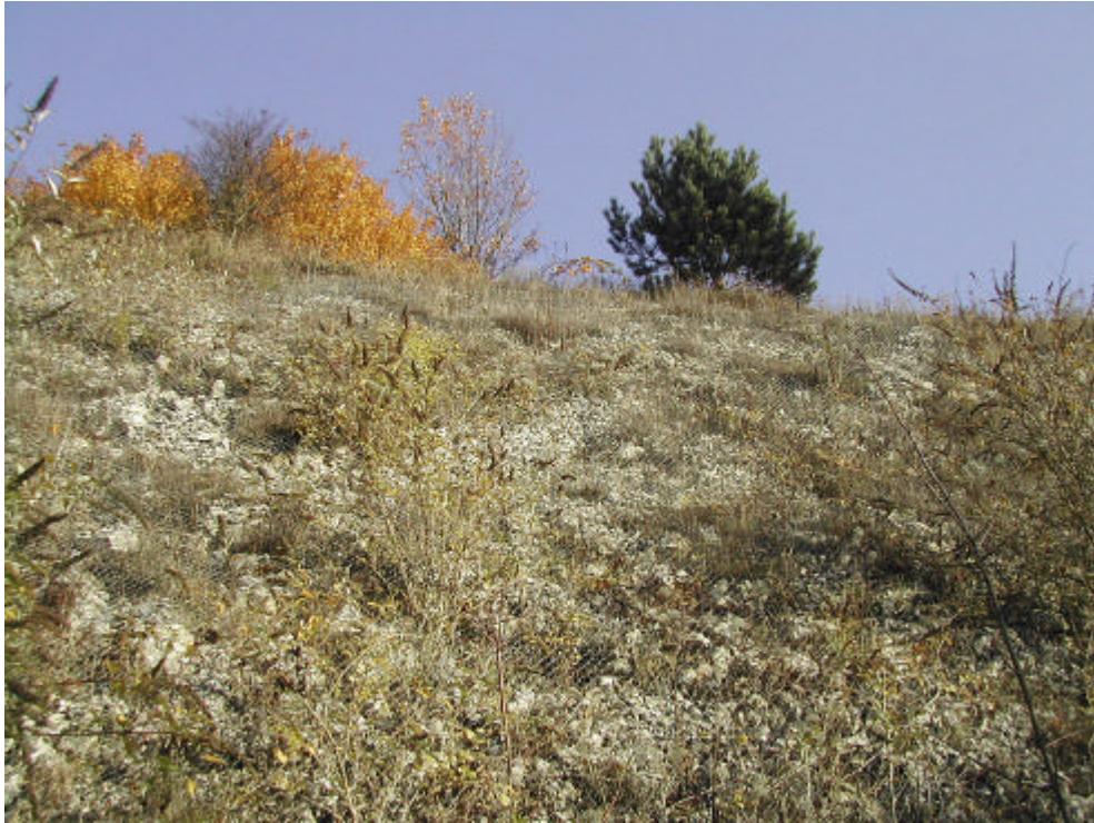
Figure 6. The Spitfire Bridge road cutting east of Winchester, a similar section to that a Black Rock. This site illustrates how rock debris and vegetation has accumulated behind the ‘mesh’ over time, completely obscuring the geological exposure. Tony Cosgrove/ English Nature.
