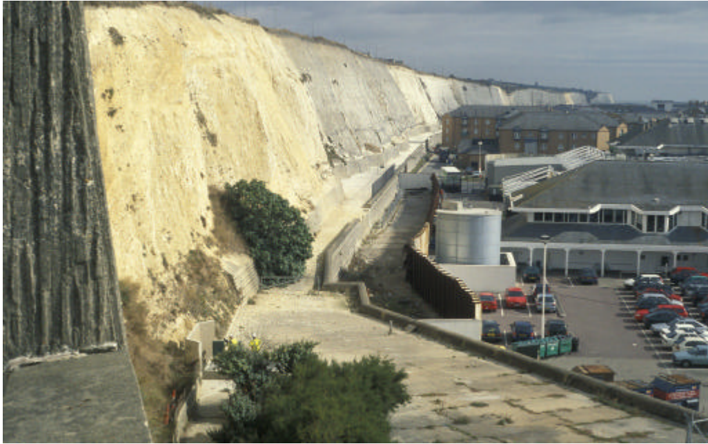
Figure 2. The cliffs at Black Rock looking eastwards. The previously 'meshed' area of chalk is clearly visible as a darker area. Colin Prosser/ English Nature.
