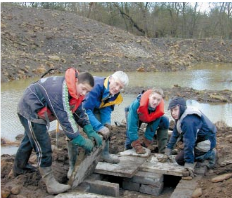
Members of a Watch group construct an otter holt at Low Barns Nature Reserve as part of the Mineral Valleys Project. Dave Long/Durham Wildlife Trust
