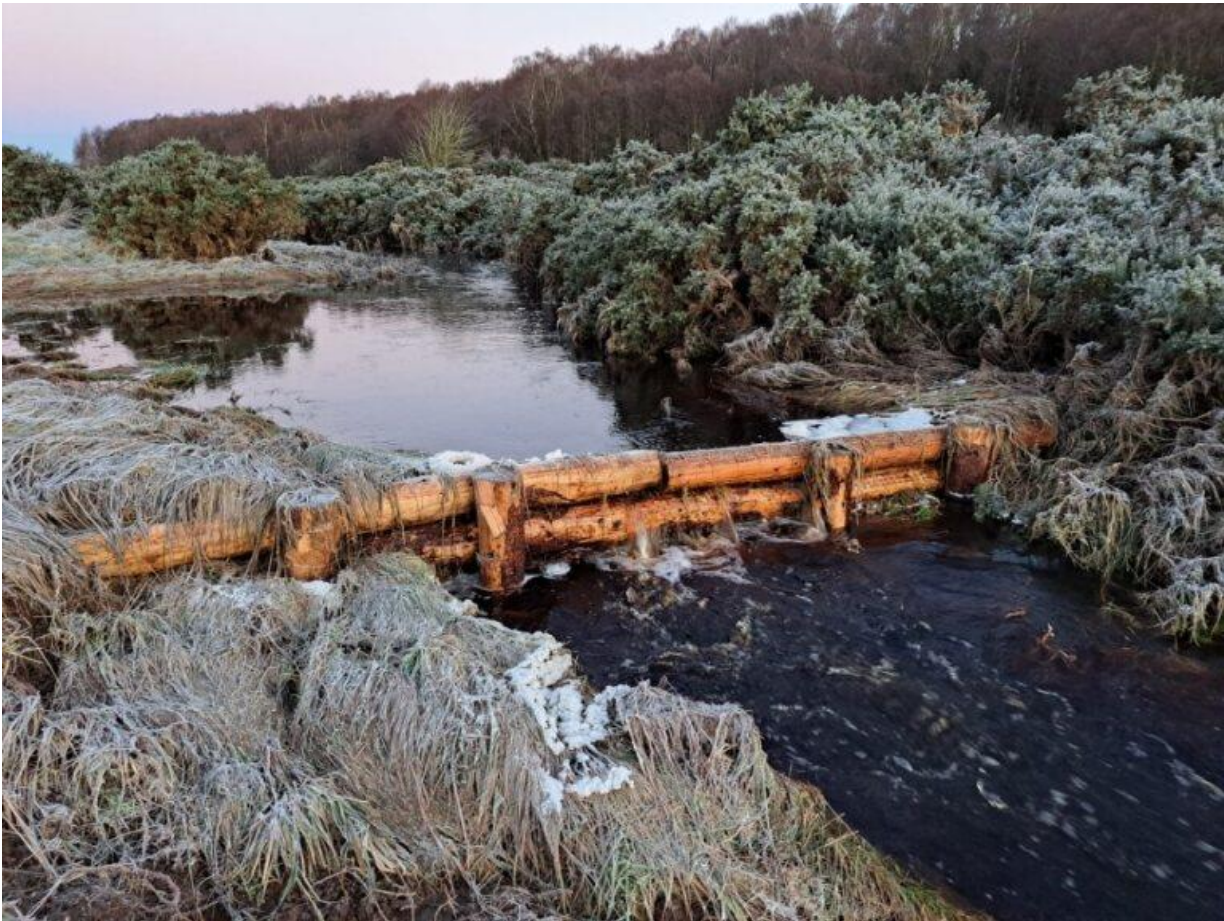
Harwood Burn leaky dam. Photo credit: Groundwork North East and Cumbria
